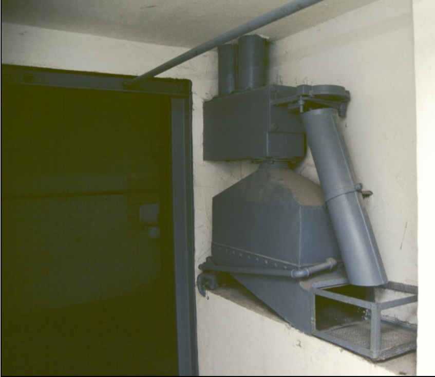
Illustration 23: The inside of one of the four Degesch delousing chambers as it can be seen today in Dachau. At the top, the can opener controlled from the outside. The Zyklon pellets slid through the pipe into a wire-mesh basket at the bottom, through which warm air was conducted by the heater/fan unit (below the can opener).
