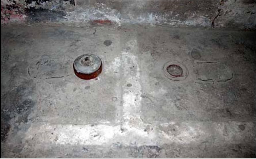
Illustration 6: Two toilet drains with imprints of the toilets and the stall walls still visible on the floor of what tourists experience as “the gas chamber” at the Auschwitz Main Camp. The toilets were added in 1944 in the wash room adjoining the morgue (aka “gas chambers”) when the building was converted to an air-raid shelter, and accidentally included in the “gas chamber” when the shelter’s partition walls were torn down by the Auschwitz Museum in 1947 during their “reconstruction.”
